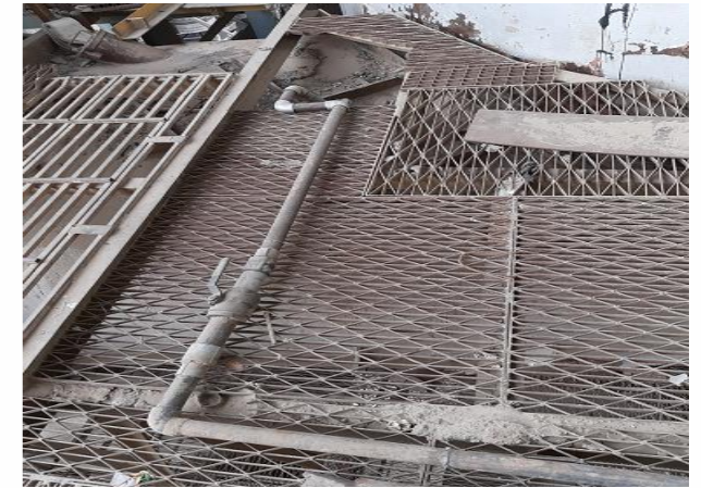
3rd feeding point of low NCV feeding point at ILC TAD duct outlet duct connecting to ILC
