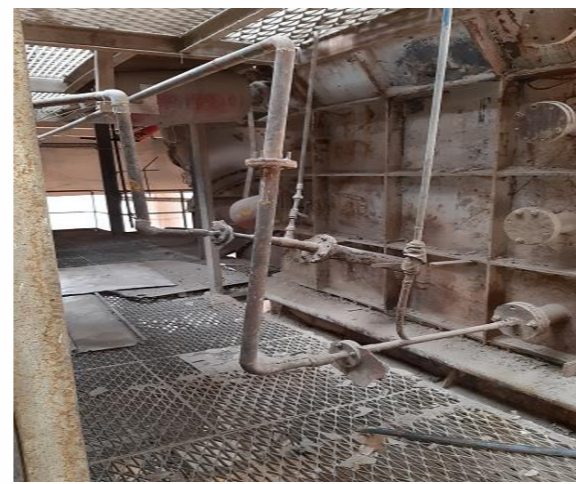
High NCV feeding point at reducing zone of calciner
