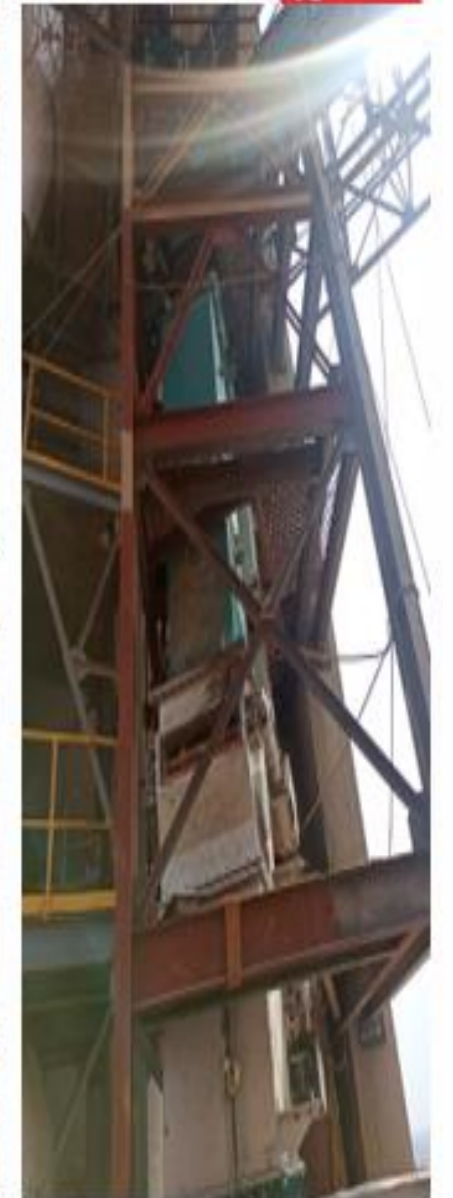
Feeding System at Preheater
