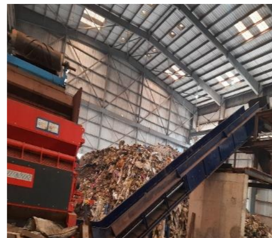
Weima Shredder installed
